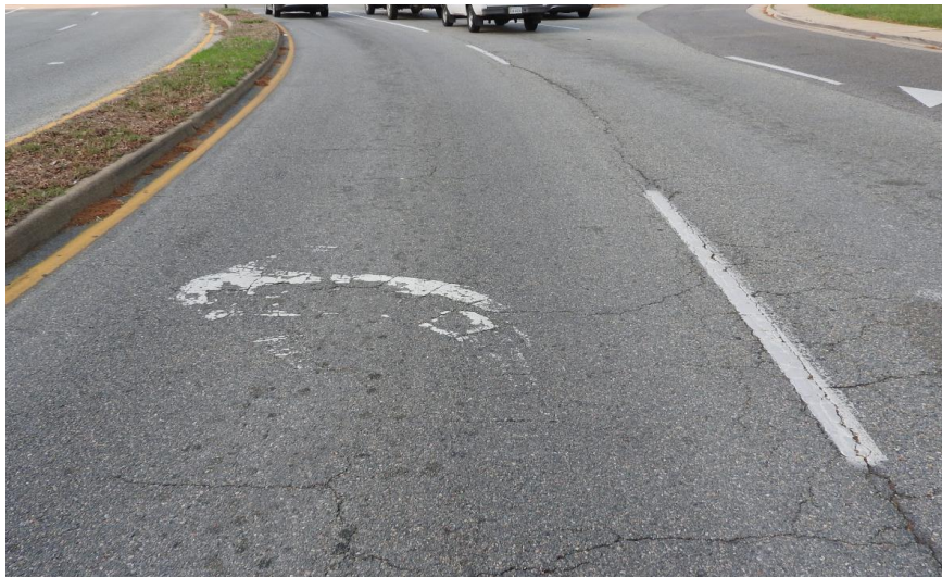
Picture 2: Asphalt Cracking and Faded Pavement Markings on Old Buckingham Rd. (SB approach)
