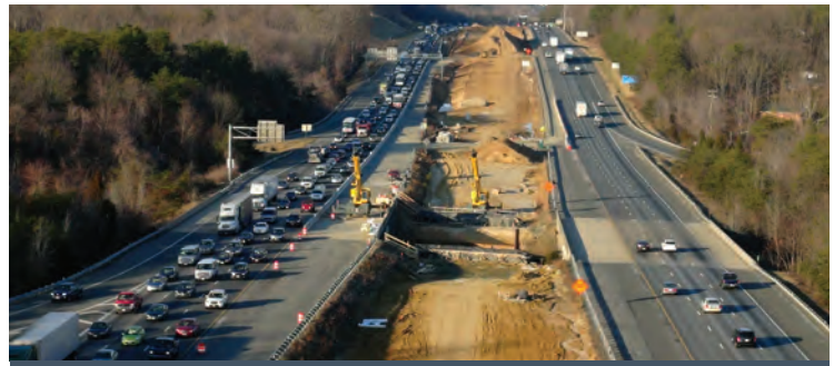
Remediation of local soils during construction of Branch’s I-95 HOT Lanes project.
