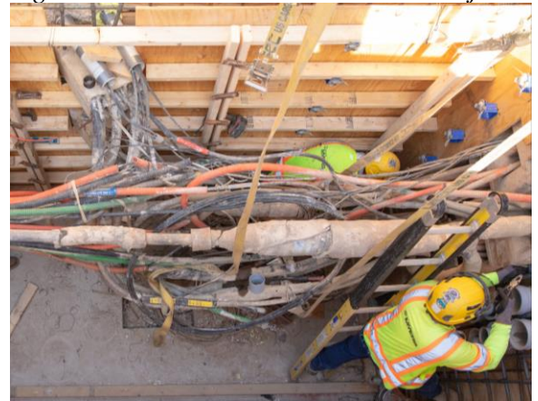
Figure 4.2: Utilities on Central Ave DB Project
