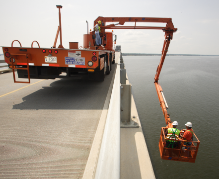
After the collapse of the I-35W Bridge in Minneapolis on August 1, VDOT ordered inspections of its 11 deck-truss bridges, which were of a similar design to the collapsed bridge. The inspections were completed in October, and no serious safety issues were found.
