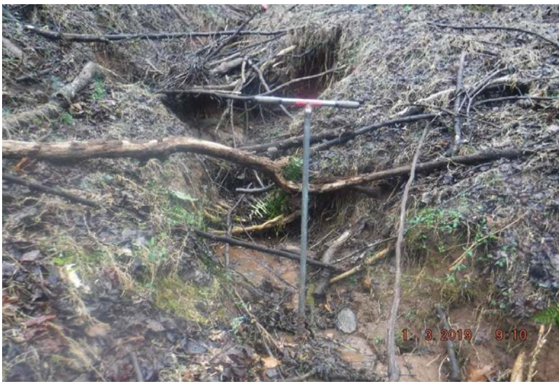
Looking upstream at Stream Reach 135-A. The reach was moderately incised with areas of active erosion. The right and left riparian buffer consisted of 100% optimal canopy cover. The instream habitat had leaf packs and substrate of various particle size but lacked riffle and pool complexes. The reach had no channel alterations.
