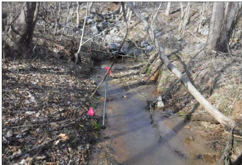
Looking upstream at Stream Reach 2-A. The reach was incised with active erosion at a culvert located at the top of the reach. The riparian buffers consist of 50% mature tree cover and 50% impervious surfaces associated with State Route 220. The in-stream habitat is present in 10%-30% of the reach and consisted of riffles, pools, leaf packs and substrate of various particle sizes. The channel was riprapped at the culvert.
