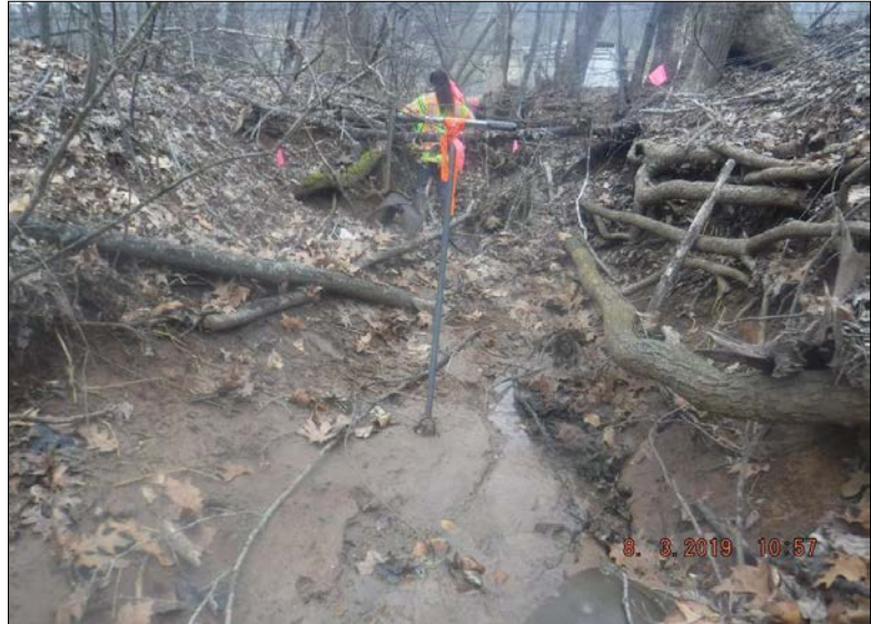
Looking southwest (downstream) at Stream Reach 63-B. Erosion is present along both banks as a result of stormwater surges, but the majority of banks are stable. Both banks' riparian buffers are primarily forested with greater than 60% tree canopy cover but contain canopy gaps dominated by dense herbaceous vegetation. Stable habitat elements are present in 10-30% of the reach. The upstream end of the reach is fed by a culvert, disrupting less than 20% of the reach.
