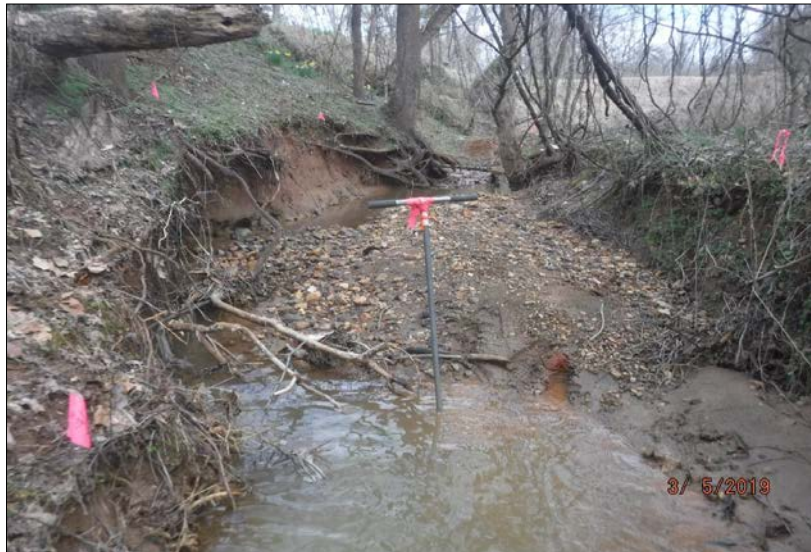
Looking downstream at Reach 7-C. The reach was frequently incised with active erosion throughout and near culverts at the top and bottom of the reach. The right riparian buffer consisted of a 90% tree cover with a maintained understory and 10% tree cover with a mature canopy. The left riparian buffer consisted of 60% tree cover with a mature canopy, 10% tree cover with a maintained understory, 10% maintained lawn, and 20% non-maintained herbaceous areas. The in-stream habitat throughout the reach consisted of riffles, pools, leaf packs and substrate of various particle sizes, however, the reach was degraded due to aggregation. The channel was riprapped and channelized at culverts.
