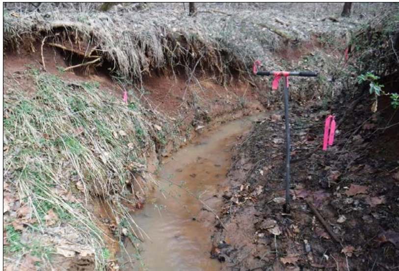
Looking upstream at stream reach 113-B. The reach had severely incised and eroded banks. The right riparian buffer consisted of 100% mature forested cover. The left buffer contained 30% mature forest cover and 70% maintained vegetation with kudzu cover. The in-stream habitat was poor, containing leaves and few pools. No channel alterations were observed.
