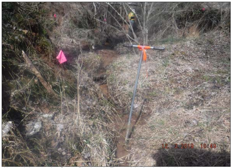
Looking north (upstream) at Stream Reach 43-A. The reach is often incised with erosion present on 40-60% of banks. The right and left riparian buffers are composed of sparse vegetation and are not maintained. Instream habitat elements are lacking and are present in less than 10% of the reach. The channel had no known alterations.
