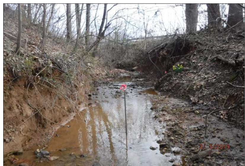
Looking upstream (northeast) at Reach 7-D. The reach was severely incised with active erosion throughout. The riparian buffers consisted of 80% mature tree cover and 20% impervious surfaces associated with State Route 220. The instream habitat throughout the reach consist of riffles, pools, leaf packs and substrate of various particle sizes, however, all habitat elements were degraded by severe aggregation. The channel was culverted under State Route 220 and riprapped at culverts.
