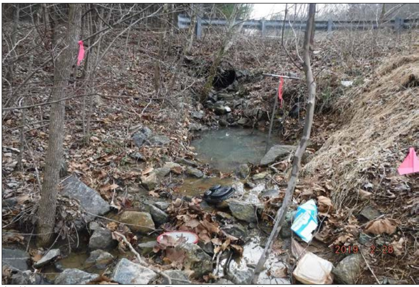
Looking upstream at stream reach 92-D. The reach had banks with some erosion and vegetation present. The right riparian buffer consisted of 20% mature forest cover, 75% mature forest with 30-60% cover containing shrub and herb layers, and 5% impervious surface. The left buffer consisted of 50% mature forest cover and 50% impervious surface. The in-stream habitat was marginal with stable elements in 10-30% of the reach. Channel alterations include rip-rap throughout the length of the reach and culverts.
