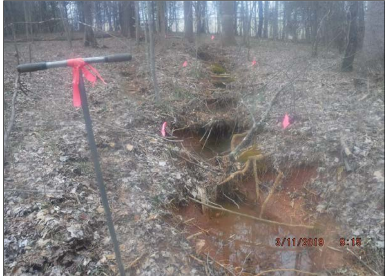
Looking northwest (upstream) at Stream Reach 67-A. The channel is often incised, with erosion present on both banks. The right bank's riparian buffer is composed largely of forest providing greater than 60% tree canopy cover, with a bit of encroachment by impervious roadway and maintained grass. The left bank's riparian buffer is composed entirely of forest providing greater than 60% canopy cover. Habitat elements are present in less than 10% of the reach. There is a culvert at the upstream end of the reach is disrupting less than 20% of the reach.
