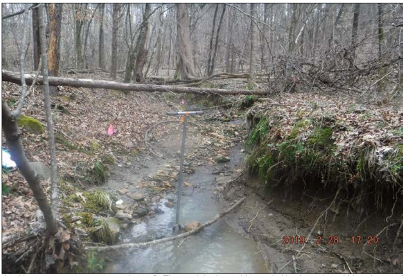
Looking upstream at stream reach 100-B. The reach had unstable, eroded banks and a cobble substrate. The right and left riparian buffers consisted of 100% mature forest cover with wetlands. The in-stream habitat contained undercut banks, woody debris and various substrate sizes. No channel alterations were observed.
