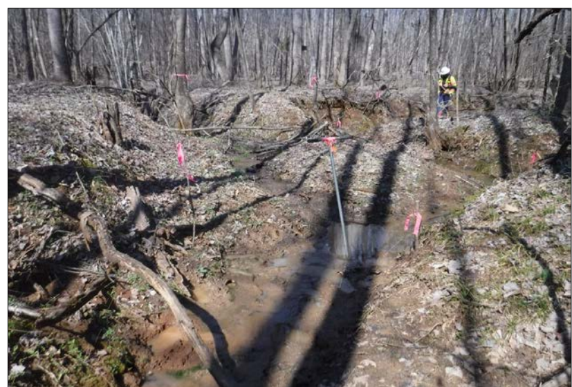
Looking upstream at Stream Reach 8-A. The reach was marginally incised with active erosion at a culvert and in a few areas of the reach. The right riparian buffer consisted of 60% mature tree cover and 40% impervious surfaces associated with State Route 220. The left buffer consisted of 90% mature tree cover and 10% impervious surfaces associated with State Route 220. In-stream habitat was present in less than 10% the reach. The channel was riprapped and channelized through a culvert.
