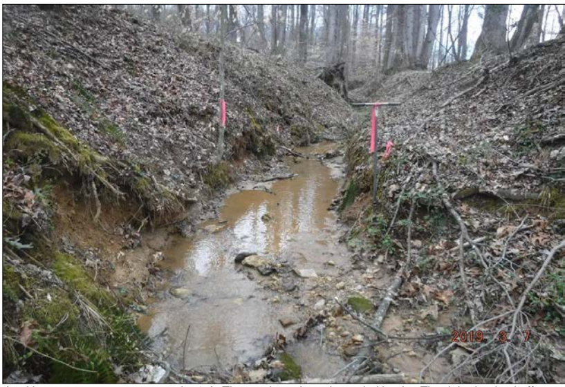
Looking upstream at stream reach 50-A. The reach moderately eroded banks. The right riparian buffer consisted of 10% maintained lawn and 90% forest with >60% canopy cover. The left buffer consisted of 10% forest with >60% canopy cover and 90% maintained lawn. The instream habitat was suboptimal with stable elements in 30-50% of the reach. No channel alteration was present in this reach.
