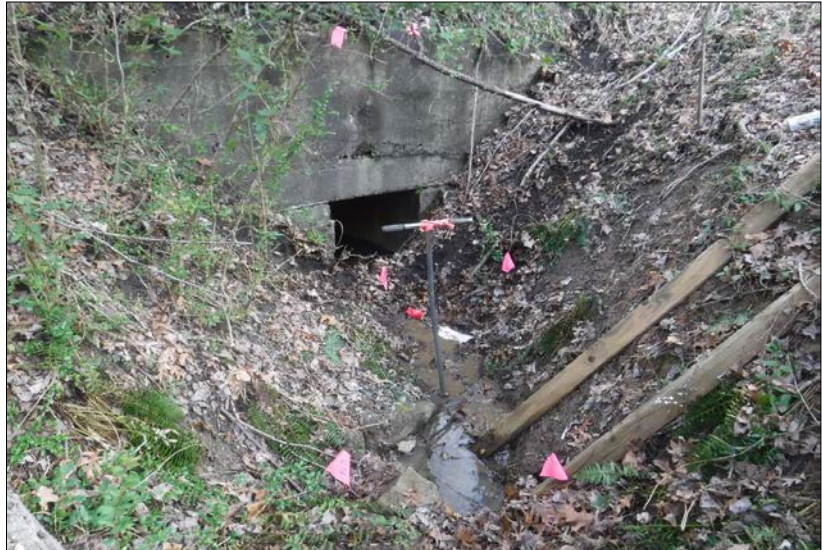
Looking downstream stream reach 42-A. The reach was marginal with areas of active erosion. The right riparian buffer consisted of 90% mature forested areas and 10% impervious surfaces associated with the railroad. The left riparian buffer consisted of 70% mature forested areas, 20% impervious surfaces associated with the railroad, and 10% maintained lawns. Instream habitat elements were less than 10% of the reach. The reach was channelized through a culvert.
