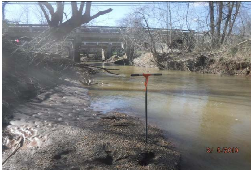
Looking downstream (west) at Stream Reach 10-B (Marrowbone Creek). The reach channel had active erosion throughout the stream. The riparian buffers consisted of 50% impervious surface associated with State Route 220 and 50% mature forest with wetlands. The in-stream habitat consisted of a deep-water with varying substrate. The channel was altered at the state route 220 bridge crossing Marrowbone Creek.
