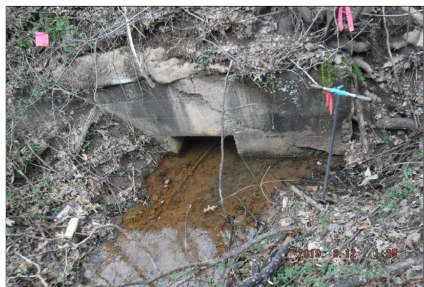
Looking downstream at stream reach 39-A. The reach was poor with frequent areas of active erosion. The riparian buffers consisted of 70% mature forested areas, 20% maintained lawns, and 10% non-maintained densely vegetated herbaceous areas. Instream habitat was present in less than 10% of the reach. The reach was channelized through a culverts.
