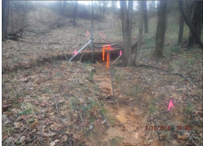
Looking northeast (upstream) at Stream Reach 69-A. The banks show areas of erosion, but vegetative protection is present along 60-80% of the reach. Both banks' riparian buffers are fully forested (>60% tree canopy cover). Habitat elements are unstable and are present in less than 10% of the reach. No channel alteration present within the reach.
