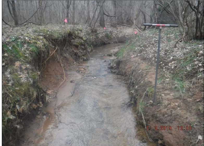
Looking southwest (upstream) at Stream Reach 75-B. The banks are slightly incised but mostly stable. Both banks' riparian buffers are forested (>60% canopy cover); a canopy gap on the right bank is occupied by dense herbaceous vegetation. Stable habitat elements are present in 30-50% of the reach. The upstream end of the reach is fed by a culvert, disrupting less than 20% of the reach.
