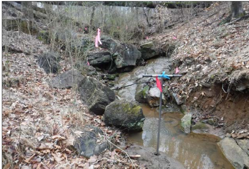
Looking upstream at stream reach 29-A. The reach channel was poor with frequent areas of active erosion throughout. The right riparian buffer consisted of 5% mature forested cover, 75% non-maintained shrub/tree layer, and 20% impervious surface associated with State Route 220. The left riparian buffer consisted of 90% non-maintained shrub/tree layer and 10% mature forested area. Instream habitat consisted of riffles, pools, leaf packs, substrate of varied particle sizes, and head-cuts, however, the reach was degraded by severe aggregation. The reach was filled in by sediment runoff associated with State Route 220.
