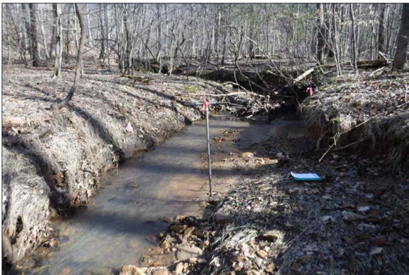
Looking upstream at stream reach 117-A. The reach had overwidened, unstable banks. The right and left riparian buffers consisted of 100% mature forest cover. The in-stream habitat was suboptimal and contained woody debris, undercut banks and various substrate sizes. There are no known channel alterations.
