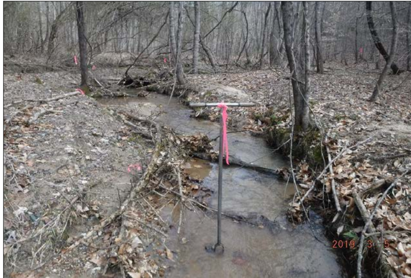
Looking upstream at stream reach 45-B. The reach had erosion present on 40-60% of banks. The right riparian buffer consisted of 98% mature forest cover containing wetlands, and 2% forest with 30-60% canopy cover containing a shrub and herbaceous layer. The left riparian buffer consisted of 100% mature tree cover containing wetlands. The in-stream habitat was optimal with stable elements in greater than 50% of the reach. No channel alterations were observed.
