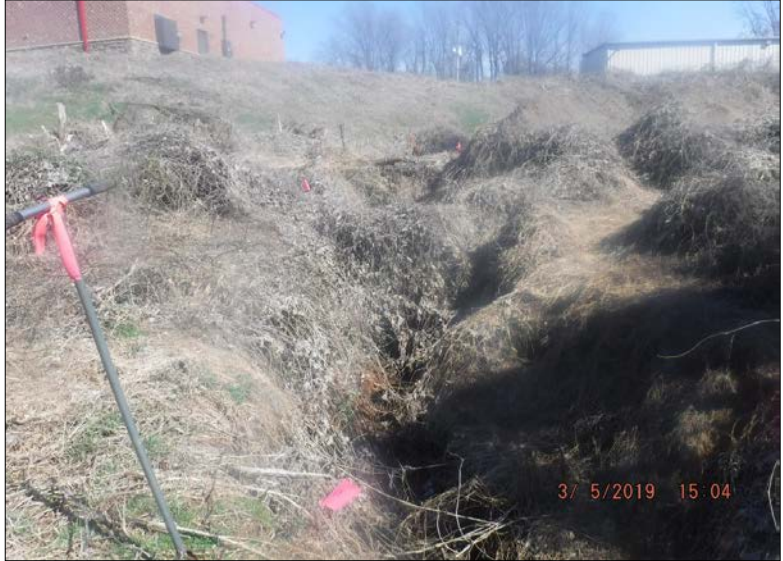
Looking east (upstream) at Stream Reach 87-A. The channel is often incised and much of the streambank is undercut. The left and right riparian buffers are covered by non-maintained herbaceous vegetation; a parking lot is adjacent to the right bank and sparse tree cover (<30% canopy cover) is present on the left bank. Instream habitat is present in less than 10% of the reach. A culvert is present at the upstream end of the reach, disrupting less than 20% of the reach.
