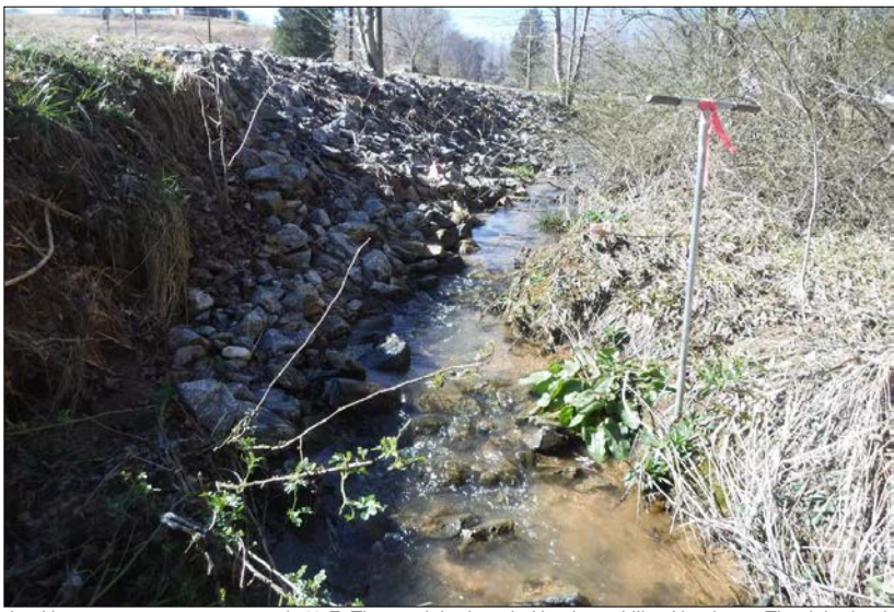
Looking upstream at stream reach 48-F. The reach had eroded banks stabilized by riprap. The right riparian buffer consisted of 80% maintained herbaceous vegetation, 2% impervious surface and 18% mature forest cover. The left buffer consisted of 85% mature forest cover and wetlands, 5% dense shrub and herbaceous vegetation and 10% maintained herbaceous vegetation. The in-stream habitat was optimal and contained various substrate sizes. Channel alterations include riprap, culverts and debris in stream.
