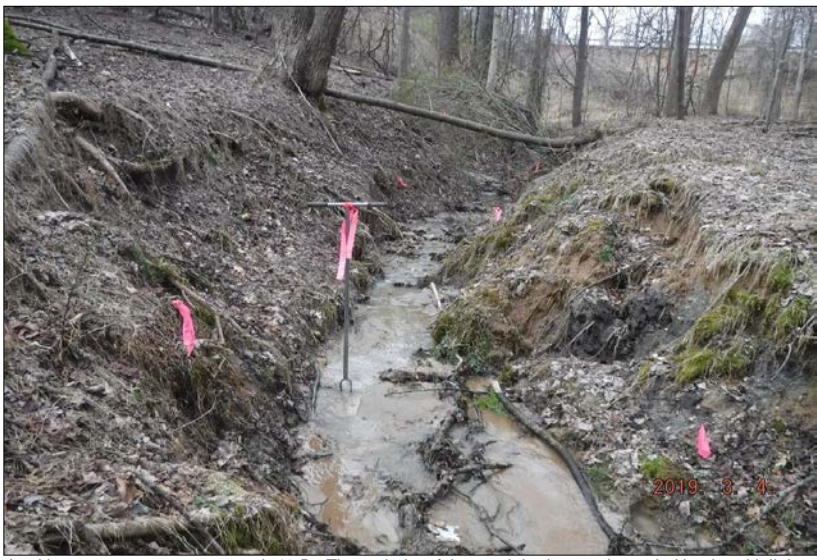
Looking upstream at stream reach 43-B. The majority of the reach had severely eroded banks with little vegetative protection present. The right and left riparian buffers consisted of 98% and 95% cover by forest with greater than 60% canopy cover, respectfully, which included fringe wetlands. The remaining riparian buffers on both banks consisted of non-maintained dense herbaceous vegetation. The in-stream habitat was suboptimal with stable elements within 30-50% of the reach, and channel alterations occurred near State Route 220.
